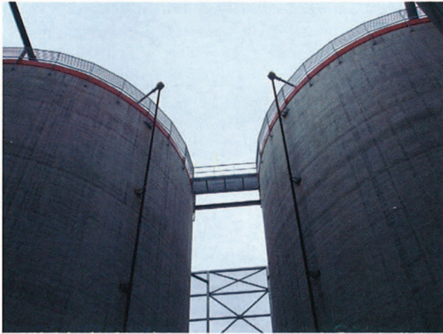
Silos fed by pneumatic transport.
